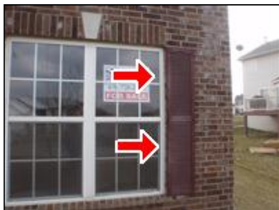
Example area, seal ALL gaped open areas around windows
